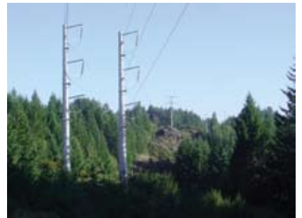
CCEC-owned transmission facilities between Gold Beach and Brookings
